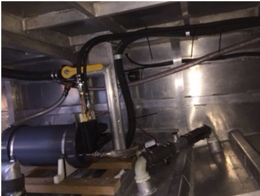
View of chiller and hoses looking aft
