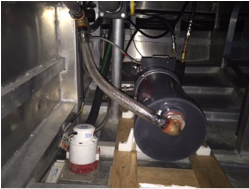
Side view of chiller and circulation pump
