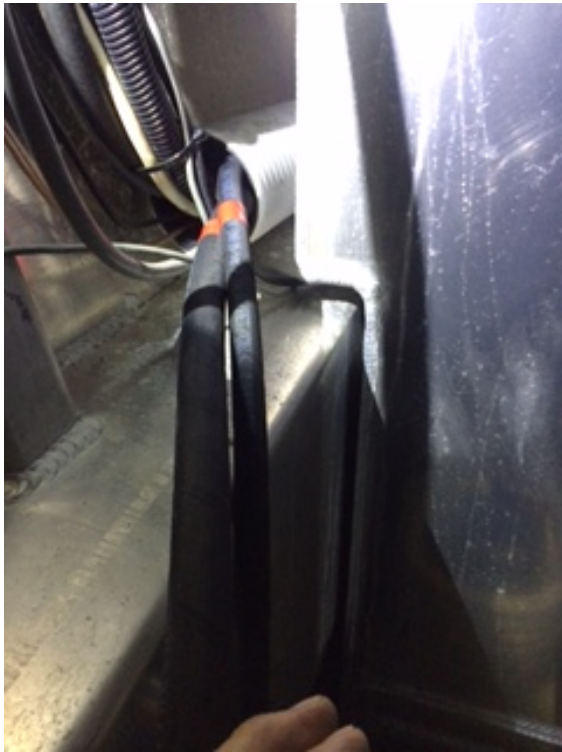
Refrigerant hoses going from engine room through duct to chiller forward of fish hold.
