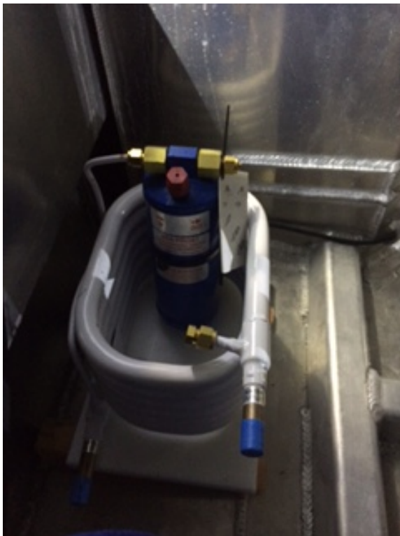
Condenser and receiver mounted in engine room
